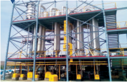
Multieffect Evaporator Vishtech CETP (Tamilnadu)
